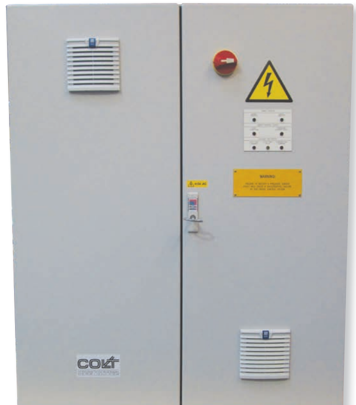
A typical Fan Control Panel with which the OPV system interfaces
