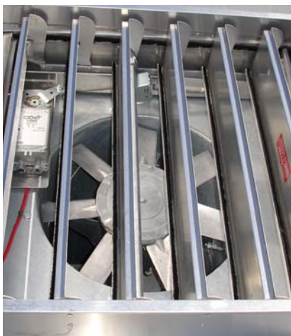
Seefire as termination piece above a fan (guard removed)
